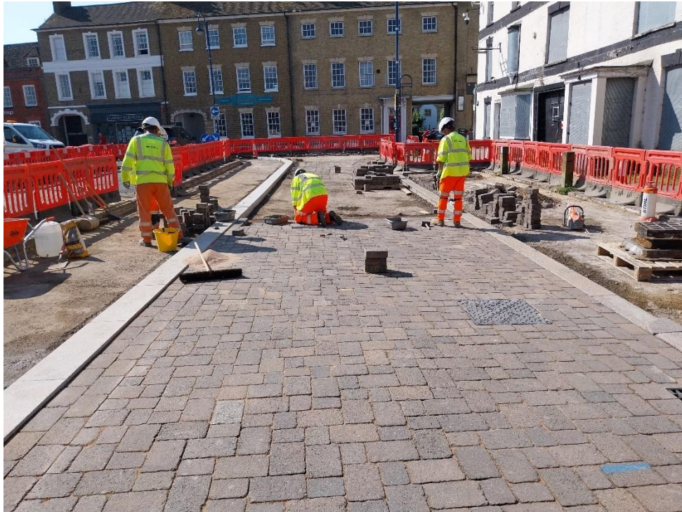
26/06/24 – Relaying of Market Place continues. New kerb line installed (left) to expand Market Square and loading bay (right) has been lifted and will be re-laid soon.
