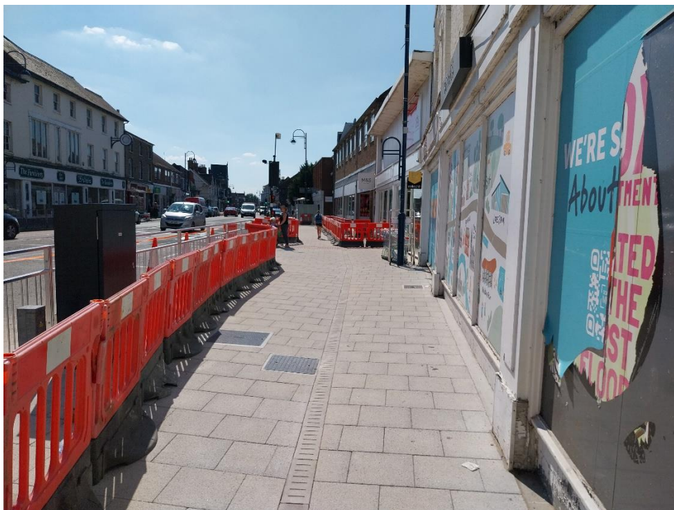
25/06/24 – Widened footway outside former Beales store nears completion. New signalled pedestrian crossing in use, pedestrian guard rail installed (right) and final areas of slab laying in progress.
