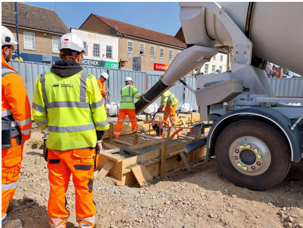
23/08/2024 – Concrete being poured for the final rain garden foundations on the north side of the Market Square.
