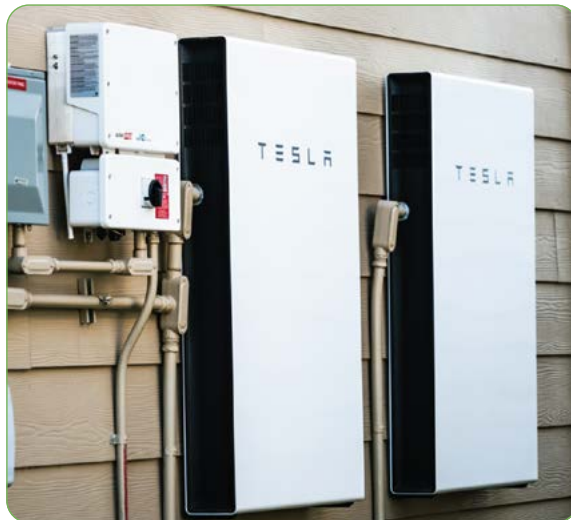
Tesla Powerwall battery system (source: www.ecoaffect.org )
