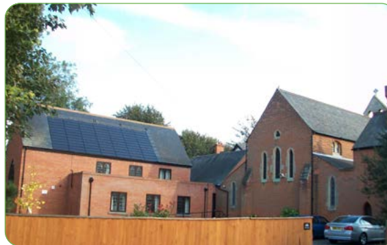
Solar panels on the rear extension of the Grade II listed Roman Catholic Church of the Sacred Heart, St Ives
