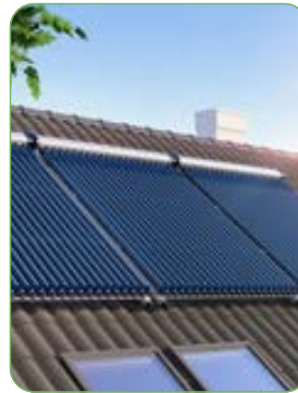
Solar Thermal Panels
