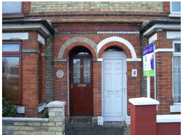
These two properties have been dealt with in very different ways which alters their character and loses the original balance and harmony between the buildings.
