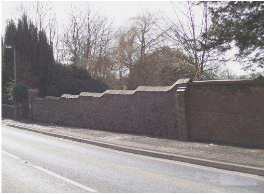
Some boundary walls are suffering from the damaging effect of poor repair with hard cement, the addition of which can lead to damage to the softer bricks.
