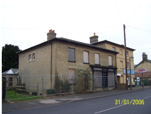
Nos 66 and 64 High Street are detrimental to the character of the conservation area in their current state
